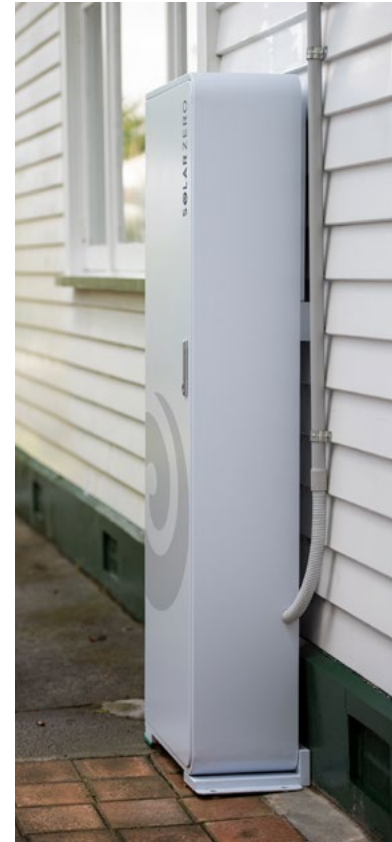
Battery storage is a critical part of a non-network, flexible distributed generation solution.
